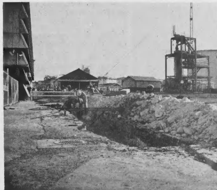
BOTH TANKS and lines were built and installed for Ethyl by the Curaçao Drydock Company and subcontractors. Even though the lead compound is almost twice as heavy as water, regular three-inch lines carry the compound to weigh tanks.
